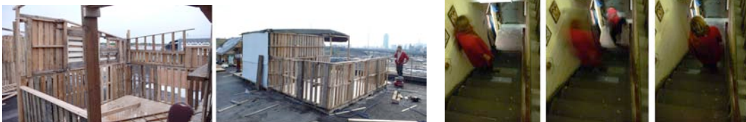
Photographs from Shantytown construction and installation in the stairwell of Flux Factory (23rd street)
